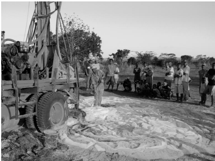
The community of Deux Baleins Nord watches as a well is drilled using foam with the converted rotary air hammer rig.
